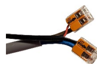
T-connector connected to Pixel cable via Wago terminal
